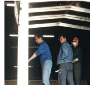
ADRIEN ROOTSAERT LED THE DESIGN & REBUILD OF THE BARGE SUPER STRUCTURE WITH ALUMINUM IN 1993. Also seen here is Wayne Rootsaert and Kent Roberts who did the welding. Photo by Keith Driver
